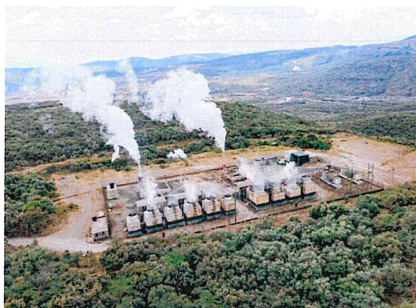
Olkaria Wellhead Generation Plants
