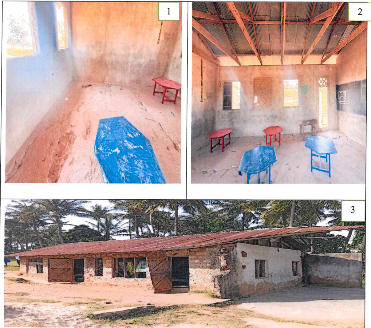
Picture 1 and Picture 2 : Showing dilapidated floors and classroom without window panes and doors at Bamba Pre-primary School, Picture 3 Showing dilapidated walls and roof at Chanagande Pre-Primary School
