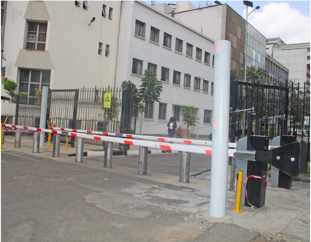
Access control equipment for security improvement
