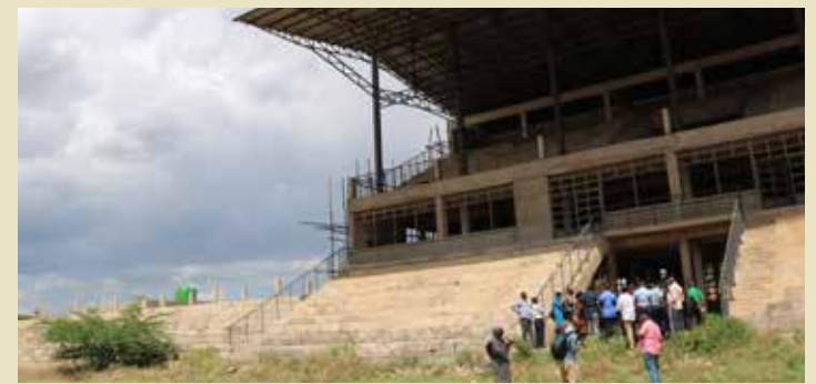
Part of Isiolo Stadium whose construction works have stalled since 2021.
