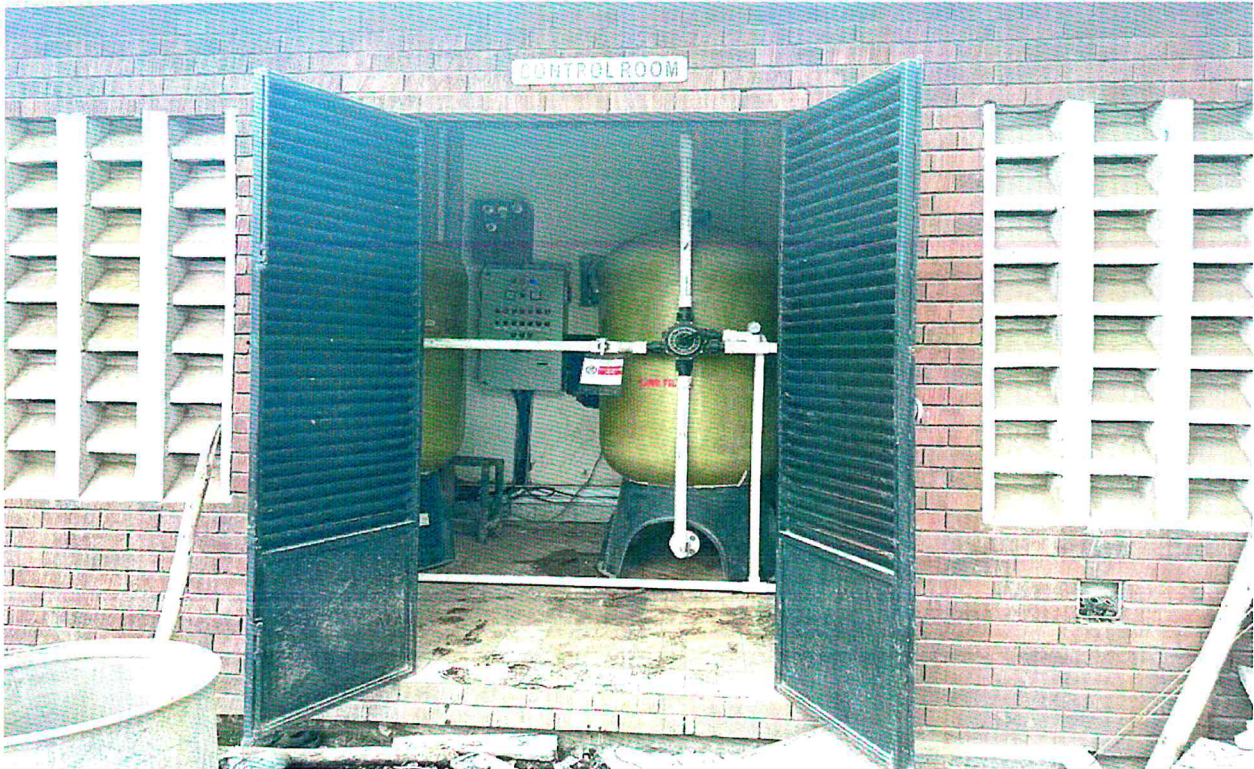
Figure 4. A modern ETP at Amalia Apartments in Syokimau
