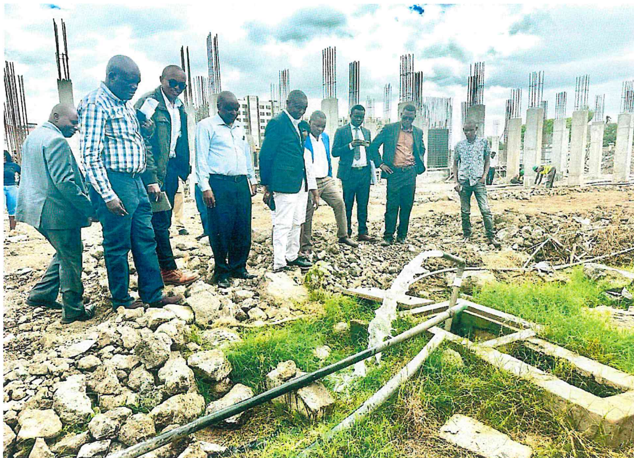
Figure 5. Members of the Public Petitions Committee accompanied by NEMA and MAVWASCO officials inspecting an ETP at Amalia Apartment
