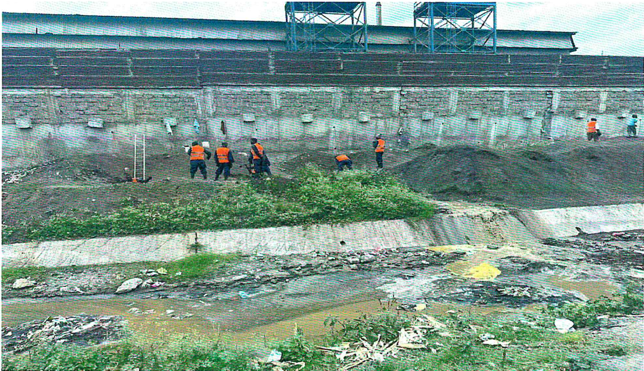
Figure 6. A sewer line operated by MAVWASCO next to Apex Steel Company in Kitengela
