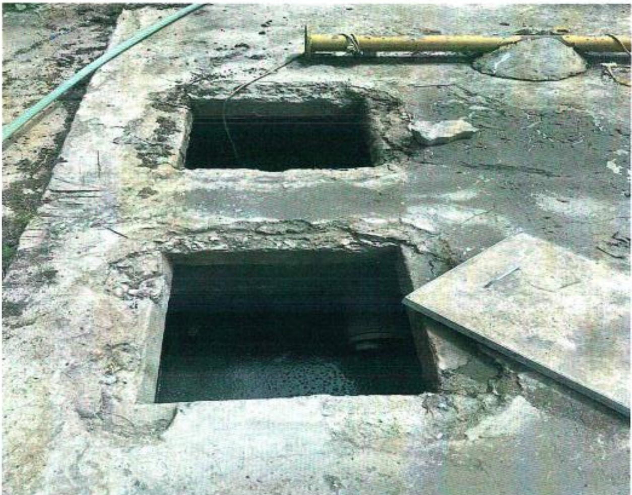
Figure 3. A dysfunctional ETP with open lids managed by MAVWASCO in Mavoko area
