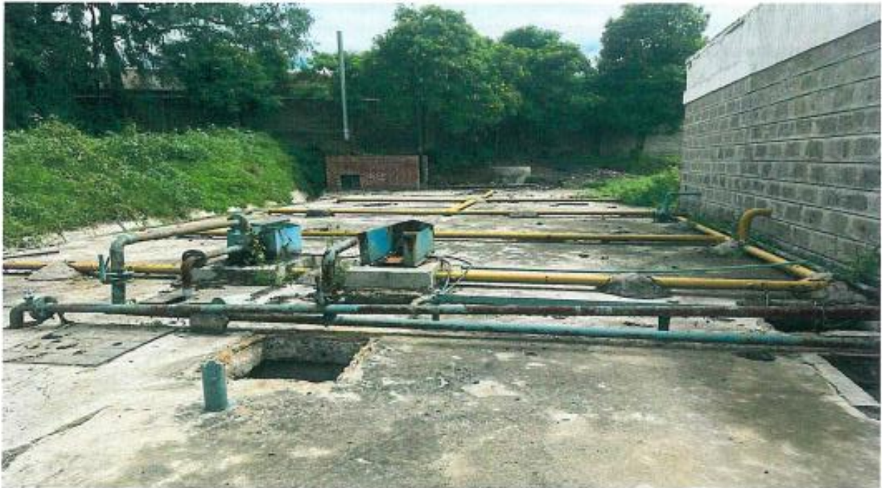
Figure 2. An Effluent Treatment Plant by MAVWASCO in Valley View Estate, Syokimau
