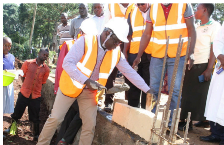
Hon. Christopher Aseka (Khwisero) laying a foundation stone for storey classrooms at Khwisero Primary School. The school is among the primary and secondary schools benefiting from the National Government Constituency Development Fund (NG-CDF).
