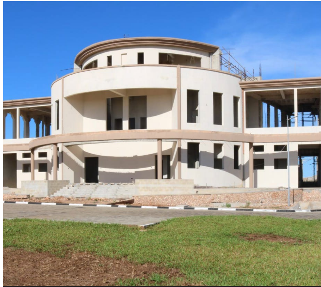
The stalled Ronald Ngala Utalii College building in Kilifi County. Tourism Committee has halted its construction over questionable funding formula.
