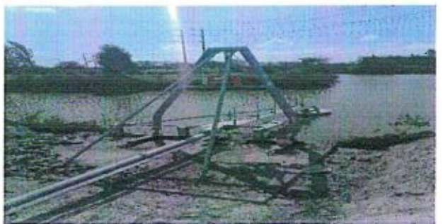
Mavoko Drinking Water Project- EAPCC _ intake
