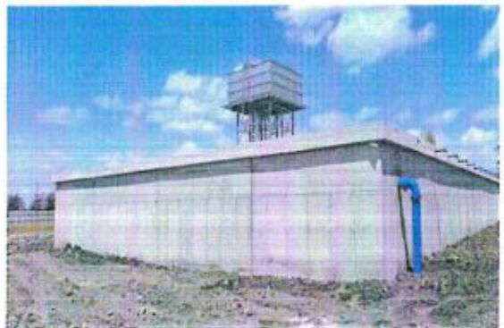
Mavoko Drinking Water Project- Syokimau_4000m3 Reservoir
