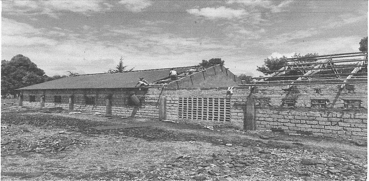
OLASHAPANI BOARDING PRIMARY SCHOOL-96 CAPACITY DORMITORY FUNDED BY NAROK SOUTH NGCDF 2019/2020 (CONSTRUCTION ONDGOING)
