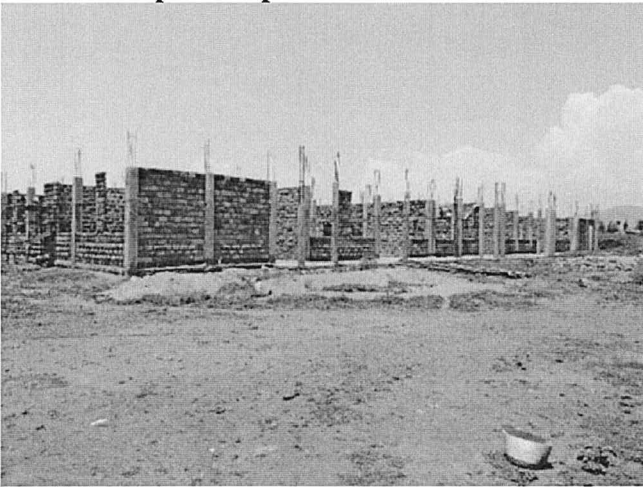
Construction of proposed Mbita technical and vocational training college at Waondo in Mbita constituency being mentored by Mawego TTI
