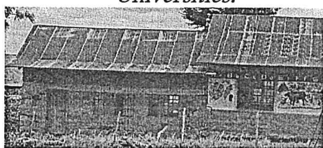
FIG 1.3: Kiamworia Primary School Deserted with bad condition of classrooms, the pupils shying off of belonging in such a school and they started migrating to far distance schools in such of better learning environment.
